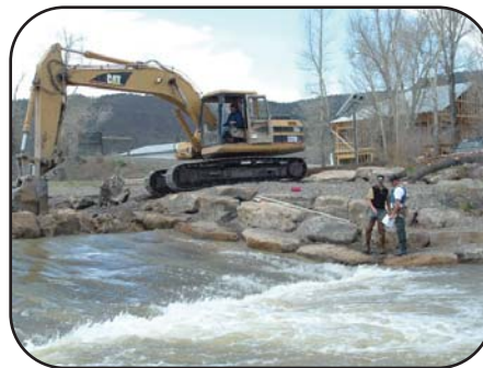
Nathan Fey and Bill Coughlin reconstruct a drop structure for the town of Ridgway.
